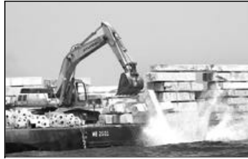
A crane pushes artificial reef material off a barge into the Atlantic Ocean off the coast of Jacksonville.
