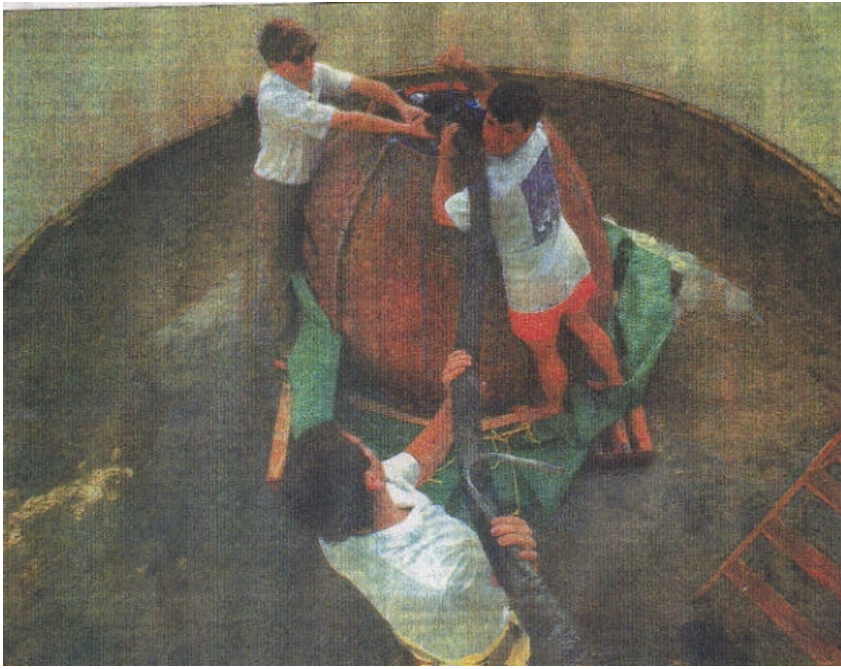
BOCA RATON- Workers pour concrete into a Reef Ball forming one of the saltwater fish tanks at the Gumbo Limbo Environmental Complex Monday. Joe Kelly (right) signals to stop the pump as Todd Barber helps fill the ball and Jim Beck (bottom) holds the hose.
