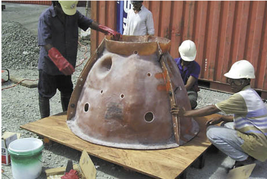
A fibreglass mould is prepared for one of the concrete reef balls.
