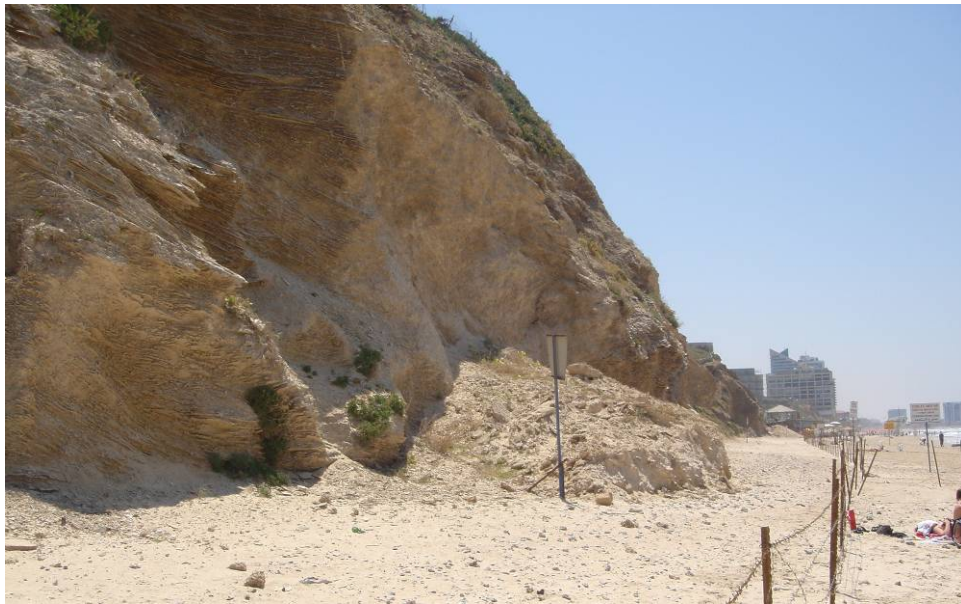
Figure 5. View of cliff erosion North of the Marina – 1 May 2007 Photograph
