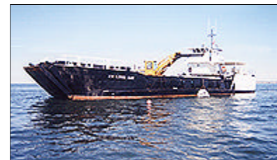
Building an artificial reef—Here workers on the R.V. Longbay lower another reef ball onto another one of the nearshore reefs in Long Bay. Note the beach in the right near background.
